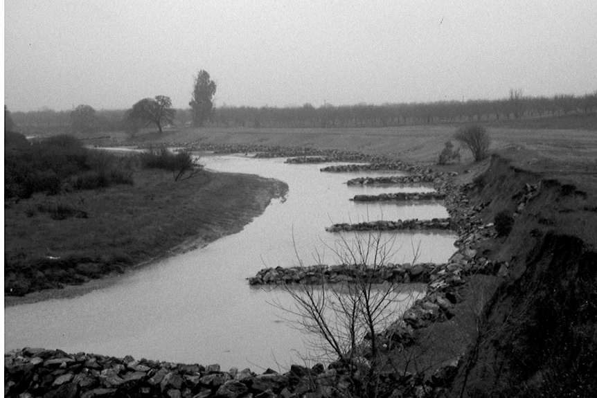
Figure 8. Even the highest flows in the winter after construction did not overtop the Bendway Weirs. Note the LPSTP is protecting the high bank in the foreground, allowing it to naturally repose.
