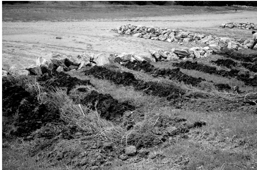
Figure 7. Composite Brush Siltation Weirs (CBSW's) were installed on the bench landward of the LPSTP in order to reduce overbank flow velocities and encourage siltation and natural revegetation.
