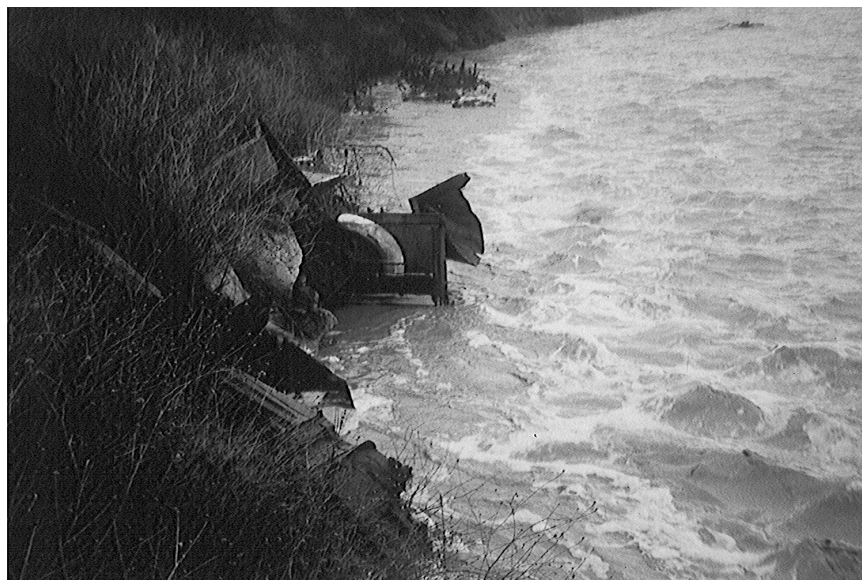
Figure 1. Erosion on the banks of Buckeye Creek was exposing waste and burn ash at the Dunnigan Burn Dump.
