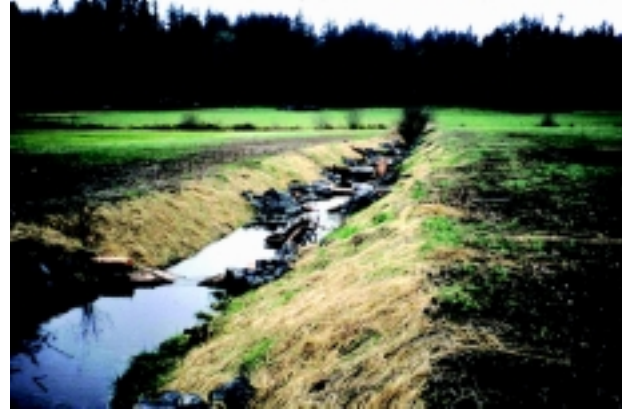
b. Bank Reshaping. Chimacum Creek, Tributary to Admiralty Inlet, Puget Sound. 1996.
