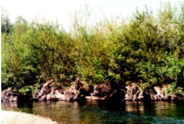
b. Log Toe with rootwads, boulders, soil-reinforced lifts and plantings. Four years after construction. Green River. 1998. Source: King County Department of Natural Resources.
