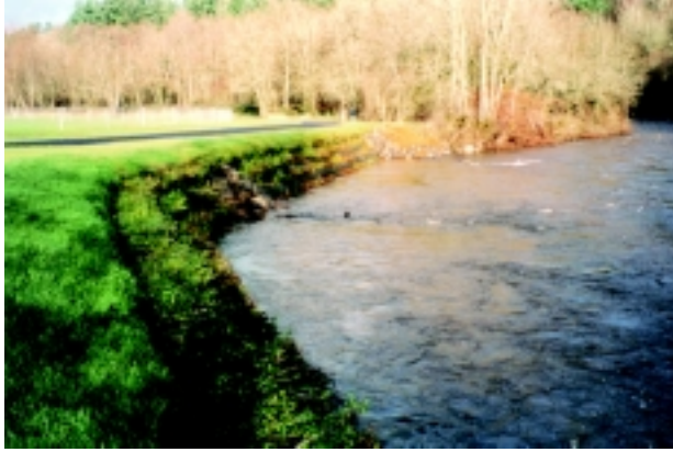
a. Soil Reinforcement lifts with barbs and rock toe. Salmon Creek, Tributary to Columbia River. 1997.
