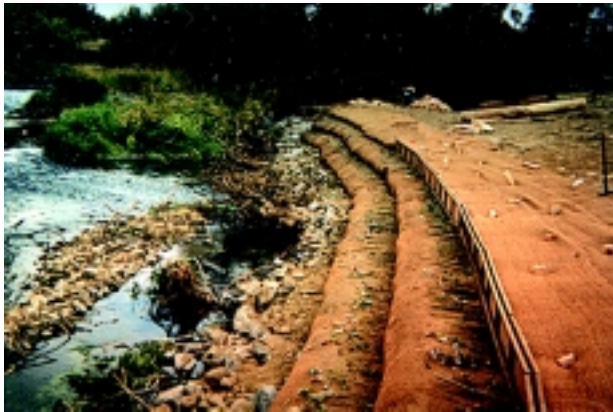
b. Soil Reinforcement lifts with log and rock toe. Salmon Creek, Tributary to Columbia River. 1997.
